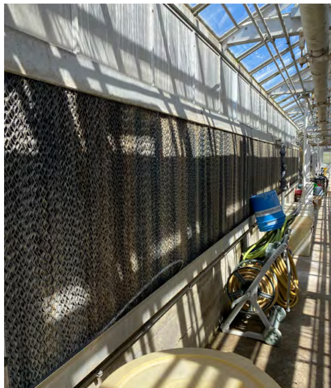
Evaporative cooling system. Photo: Andrew Demetri
